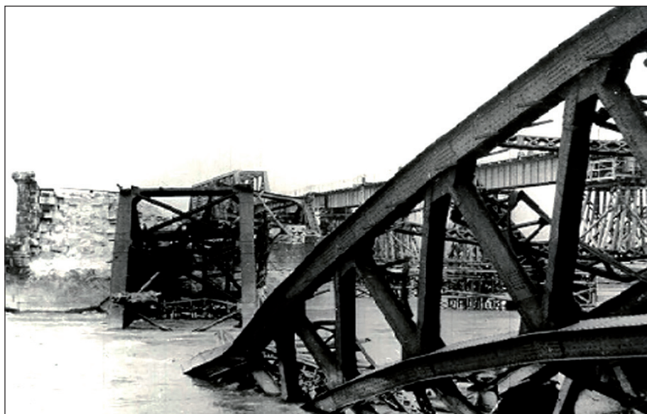
The Southern Railway Bridge in ruins
